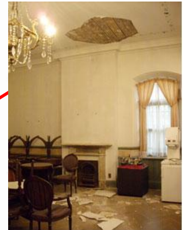
Fallen ceiling plaster at Café Abeille
