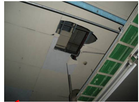
Fallen ceiling tiles
